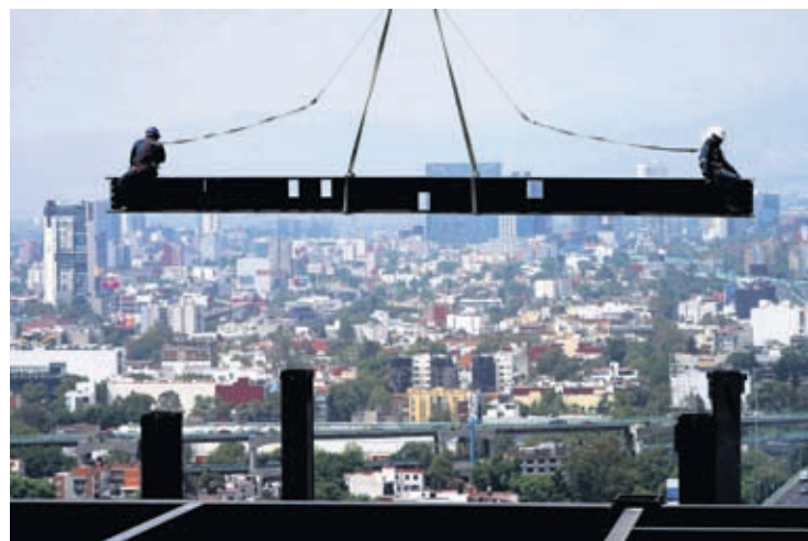
Construction workers ride on a beam hanging from a crane at the construction site of a residential high rise building in Mexico City, June 17, 2022.
